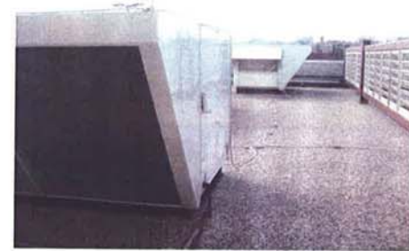
Figure 18. Roof top units
